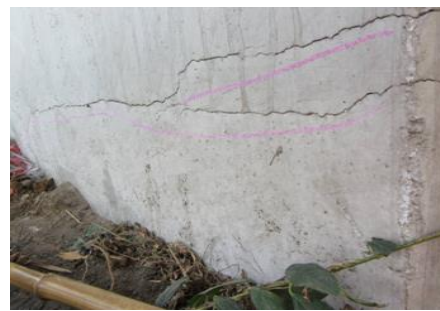
Fig. 5 – Bridge pier cracks
