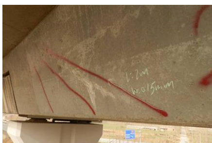
Fig. 2 – Diagonal cracks in web
