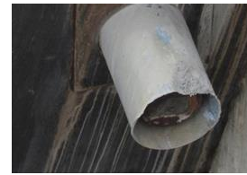
Broken protective tube
