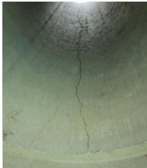
Fig. 2 - The initial bottom crack in pipe subjected to the three-edge bearing test.
