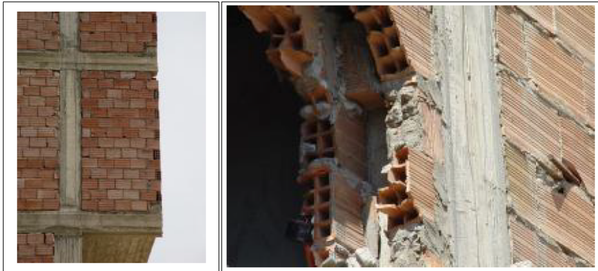
Fig. 1 – Rigid connection, BOUMERDES earthquake of May 21, 2003
