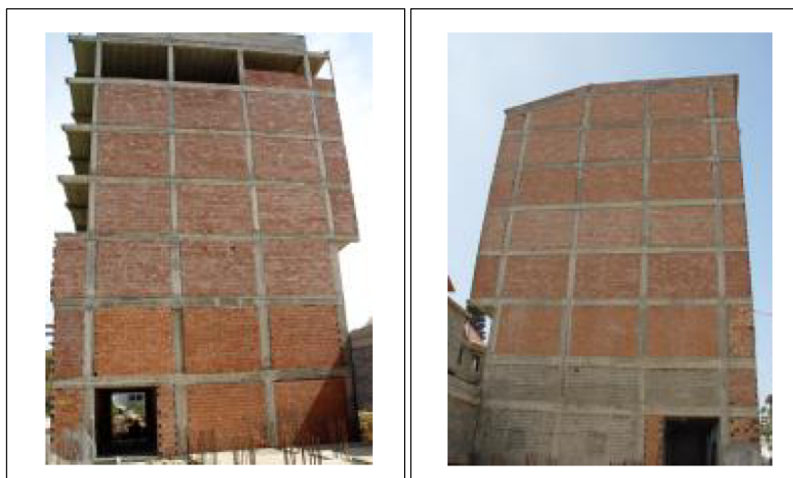
Fig. 2 – Chained masonry, BOUMERDES earthquake of May 21, 2003
