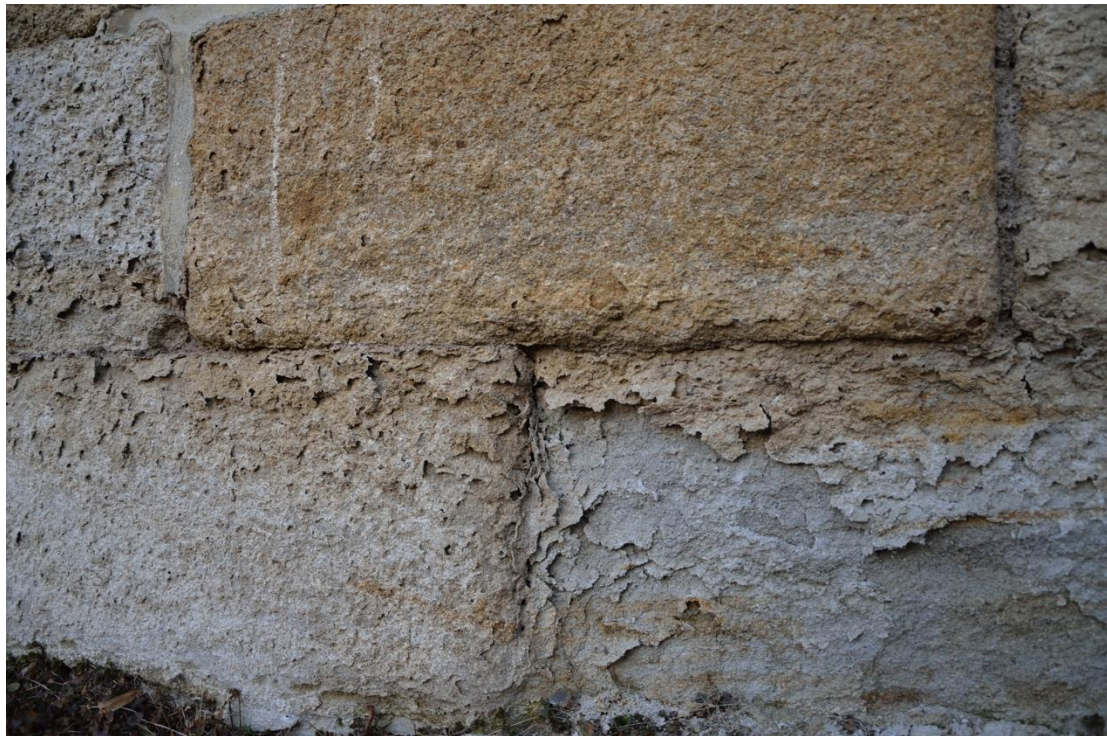
Fig. 1 – Blistering of sandstone surface with the subsequent surface scaling with strongly damaged tool traces, St. Jacob's Church, Srbeč.
