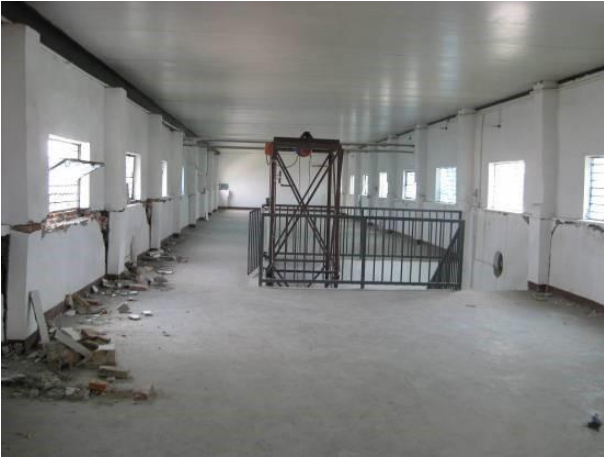
(c) Transverse cracking failure of the brick column
