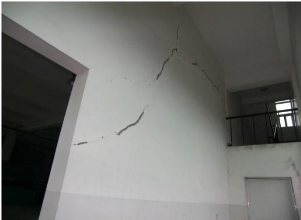
(d) Cracking and damage at the door opening
