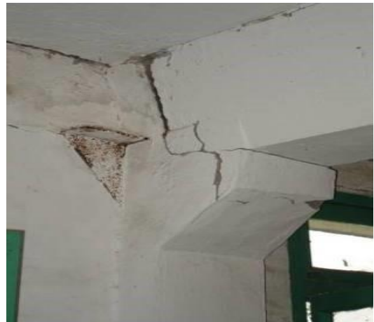
(f) Crushing cracking failure of corbel end
