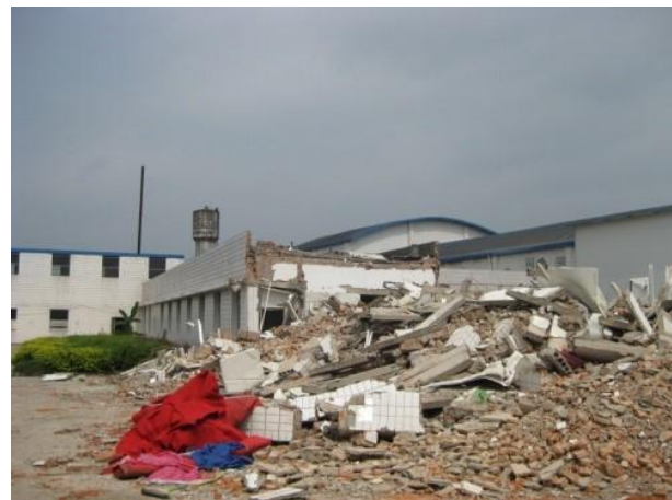
(b) Collapse of MS industrial building
