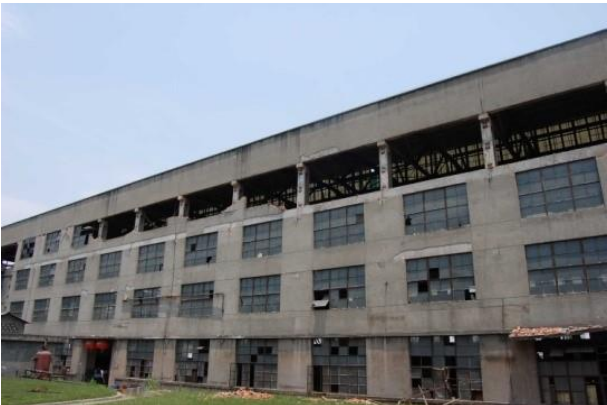
(e) Collapse of upper maintenance wall
