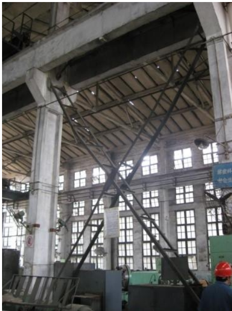
(a) Buckling of X-brace
