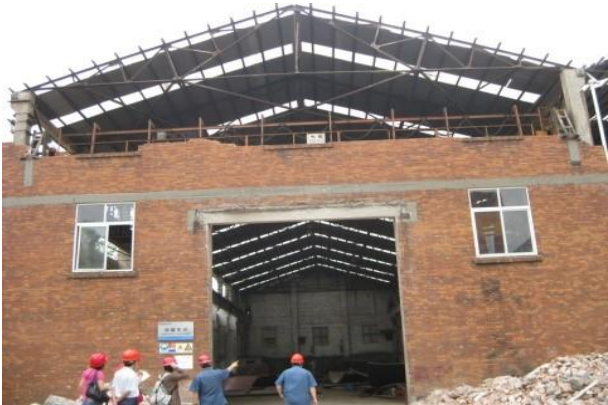
(f) Partial failure of upper maintenance wall
