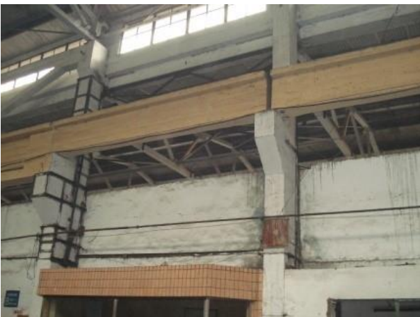
(g) Longitudinal displacement of crane beam
