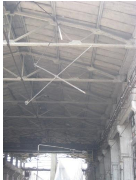
(b) Failure of horizontal contact
