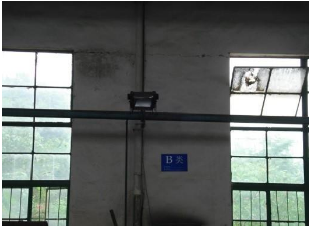
(a) Cracking of wall between windows
