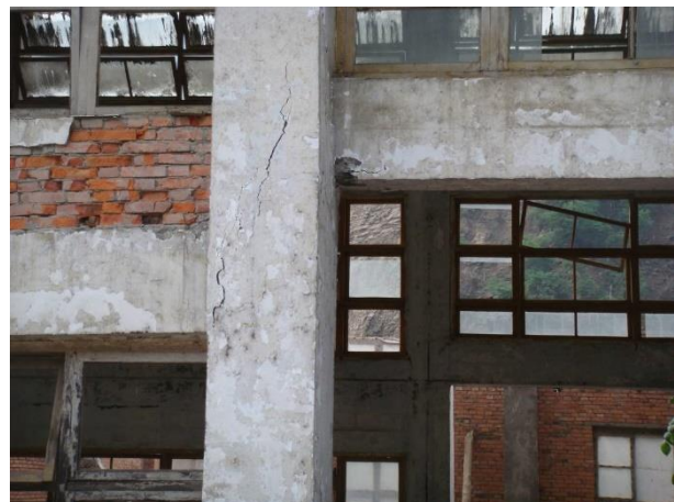
(b) Oblique cracking failure of RC frame column
