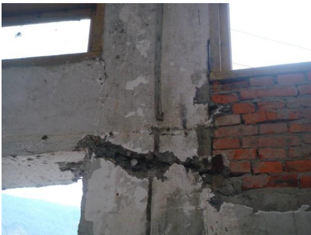
(a) Cracking failure of the RC column head
