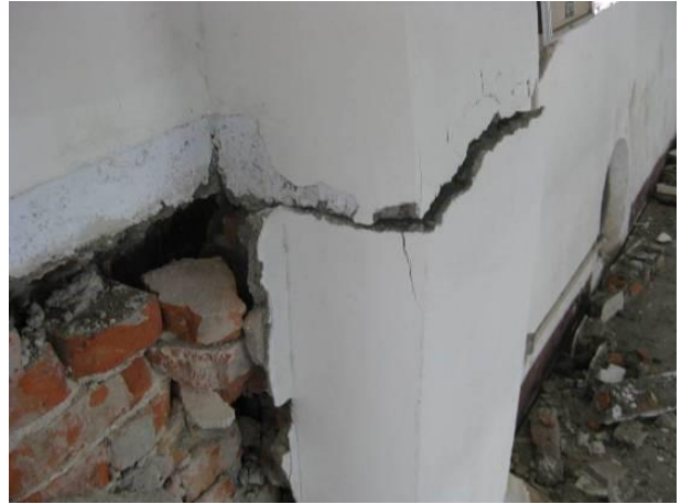
(d) Cracking failure of the lower part of the brick column
