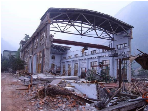
(a) Failure of Maintenance wall (gable)
