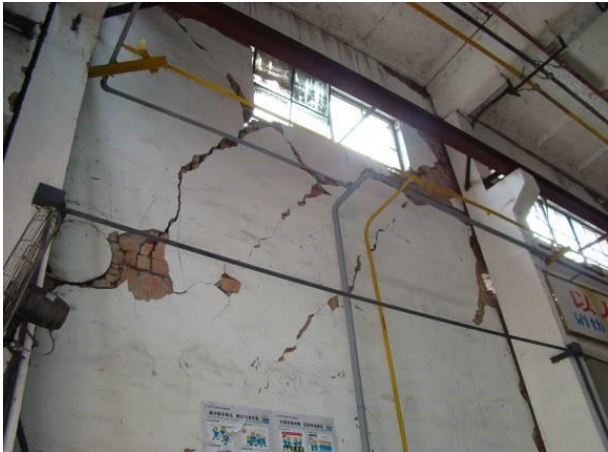
(b) Oblique cracking of wall
