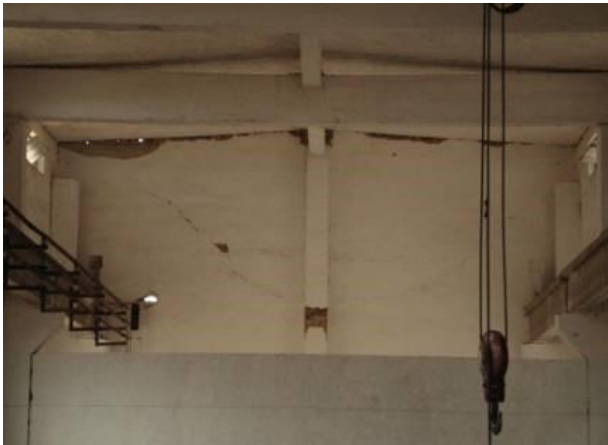
(c) Cracking of inner wall
