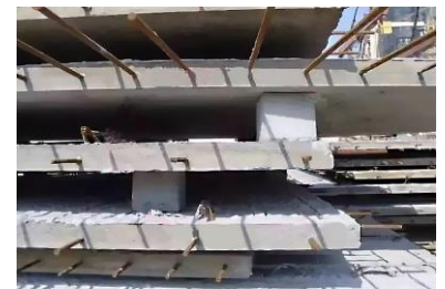
(c) Unsuitable pad position
