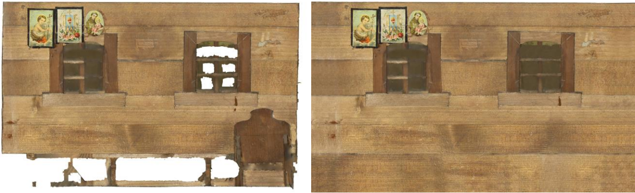
Fig. 8 – Corrections to the orthogonal projection of one of the walls, "before" (left) and "after"
