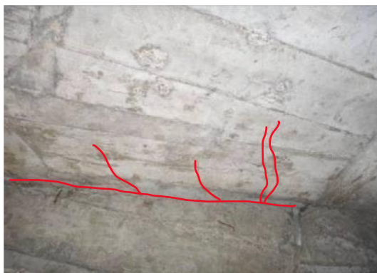
(a) Inclined cracks of tooth plate of No.11 box ( L=0.52m \delta=0.2mm )
