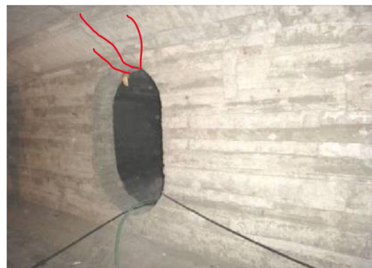
(b) Cracks in diaphragm of No.12 box ( L=1.43m \delta=0.3mm )
