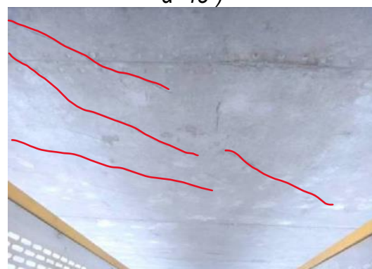
(e) Inclined cracks of the bottom plate in No. 10 hole ( L=4.4m \delta=0.3mm \alpha=45^\circ )
