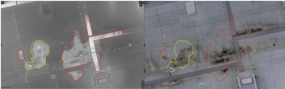
Fig. 2 – Flat roof leak sample
