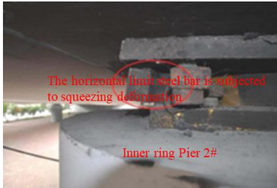
Fig. 6 – Compression deformation of lateral restraining steel bar
