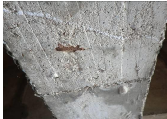
(b) - Concrete deterioration
